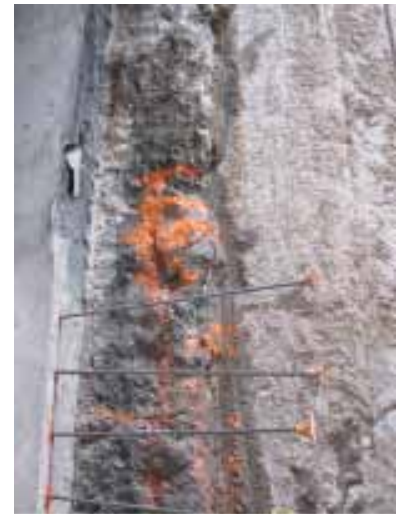
Tunnel wall (with low-strength fill) in the water table before pouring concrete wall.
